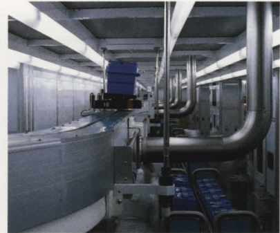
In many Intel plants, monorail systems transfer loads of wafers between production stations, speeding production and increasing efficiency and yields.
