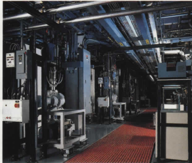
The infrastructure needed to run a fab is buried in the sub-fab level, below the vibration-resistant floor of the clean room. Stainless-steel piping and other channels deliver natural gas, chemicals, clean water and electricity to the manufacturing equipment.
